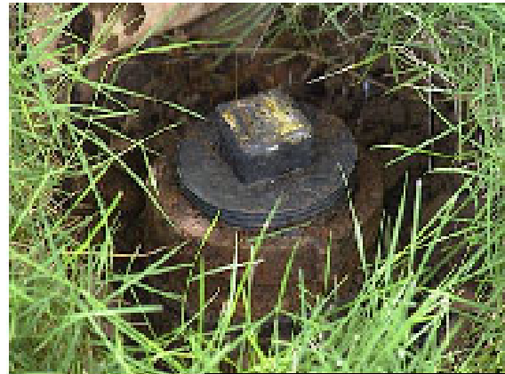
Typical sewer cleanout with properly installed plug.
